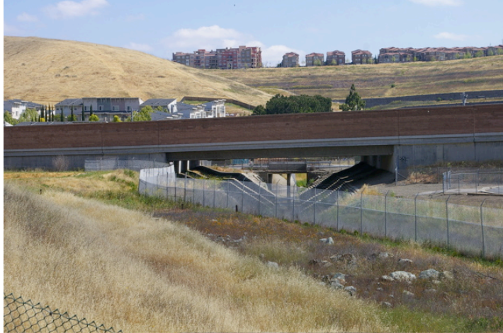
Failed mitigation: Never maintained.
